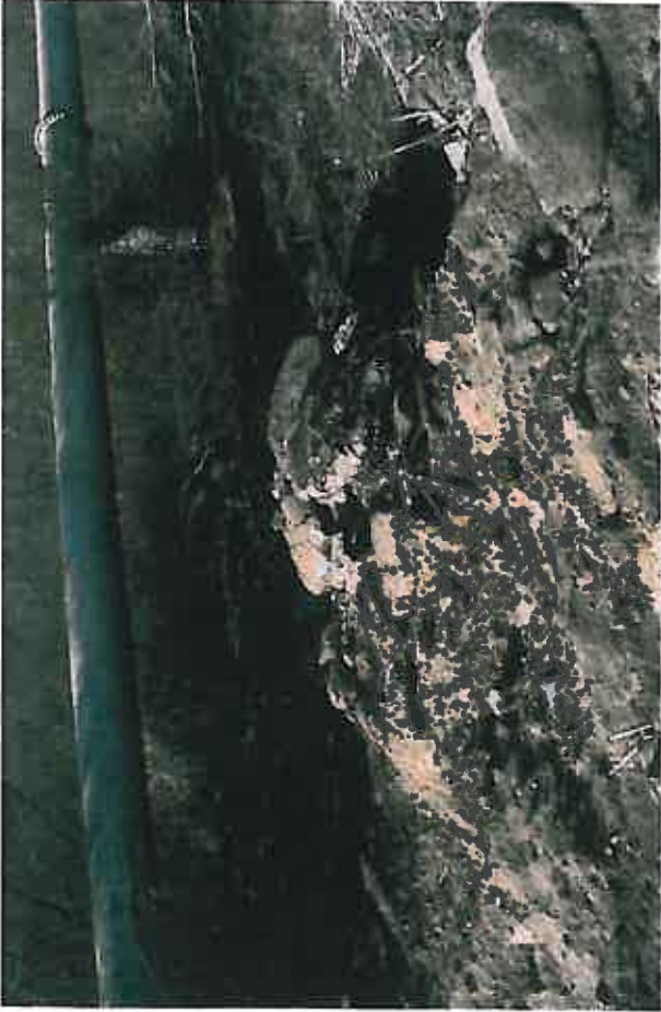
13. Concrete construction debris in the river on the northwestern portion of the Property.
